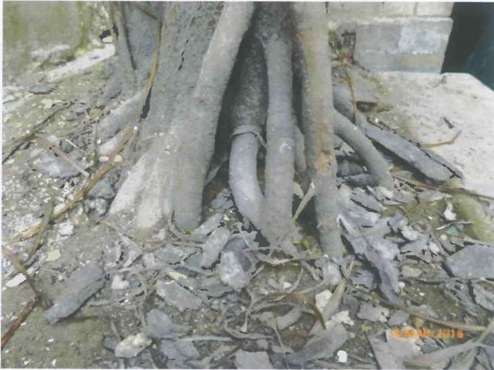
Fig. 2 Root collar is normal. Cleanliness of the planter is acceptable.
