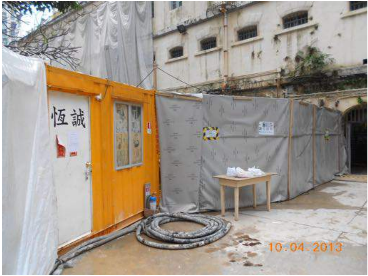
Figure 2 – Noise barrier for air compressors near Block 14
