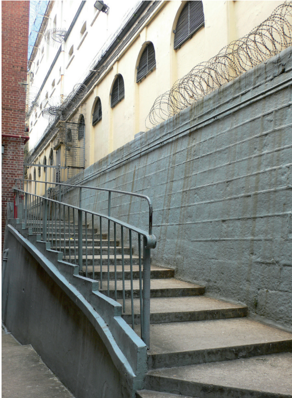
The rampted staircase giving access from one terrace to another, located between C Hall to the north and D Hall to the south
