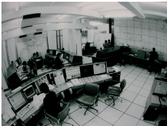
Radio Control Room
