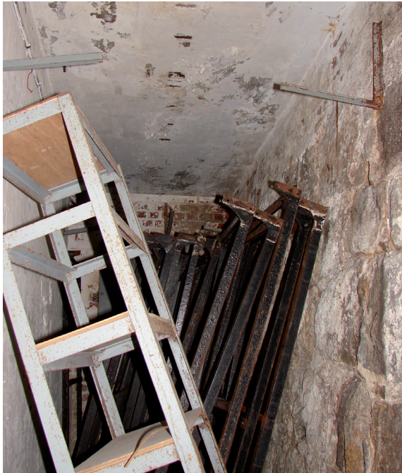
Ladder store with blocked archway
