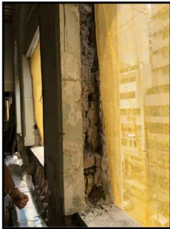
Figure 6b: Example of vertical cracks revealed after removal of rendering at a column in the east wing of the MIQ Building
