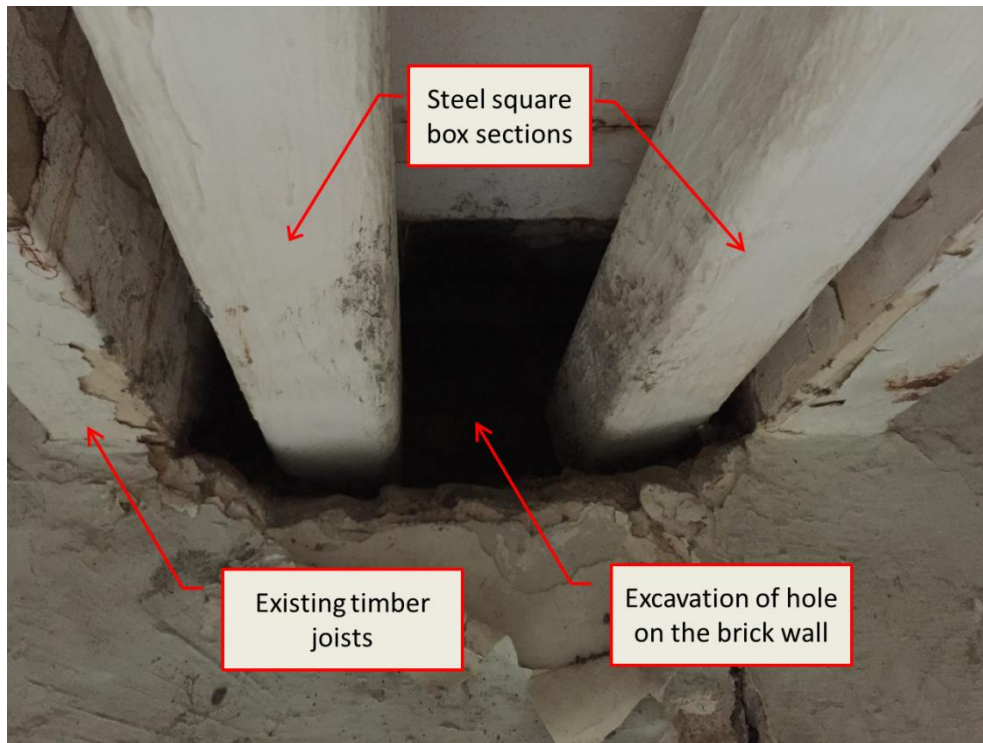
Figure 5c: Photo taken after the incident showing holes excavated in the North Wall
