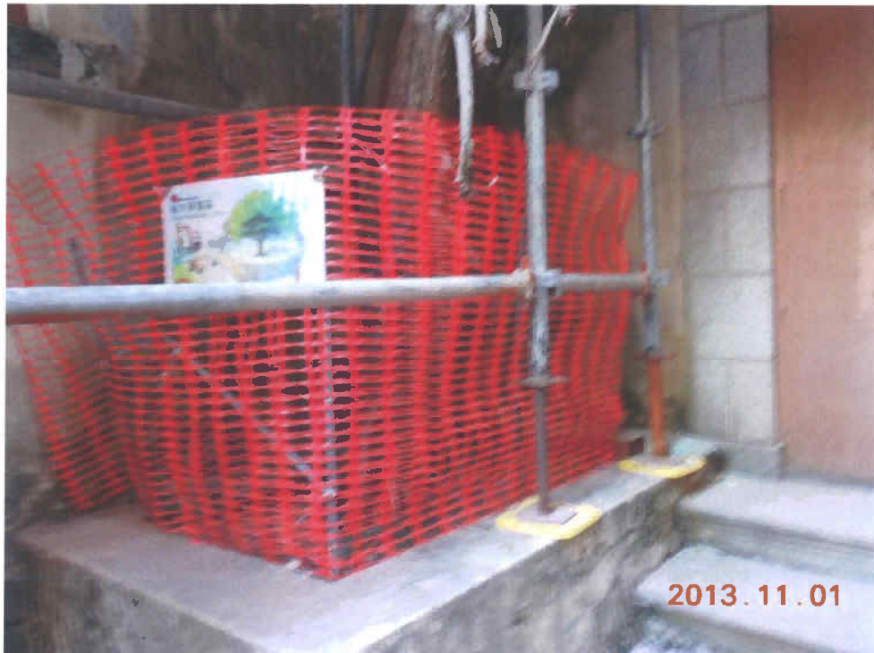
Fig. 6 The scaffold is still set up near the tree for renovation work.
