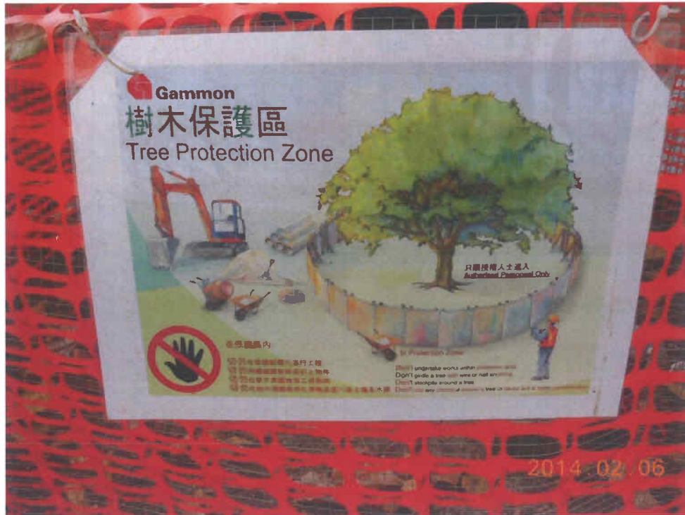
Fig. 8 Appropriate notice displays in front of the small cordon zone.
