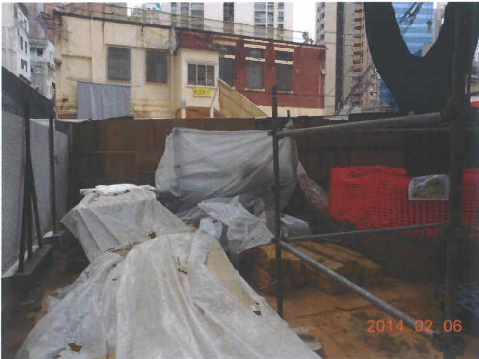
Fig. 3 Heaps of large construction materials are placed near the planter but cause no disturbance to the tree.
