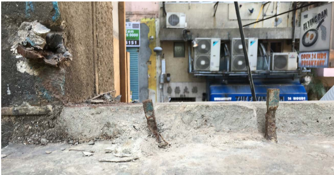
Above, photograph taken on 25 th January 2016, showing the balusters of the fence was cut.
