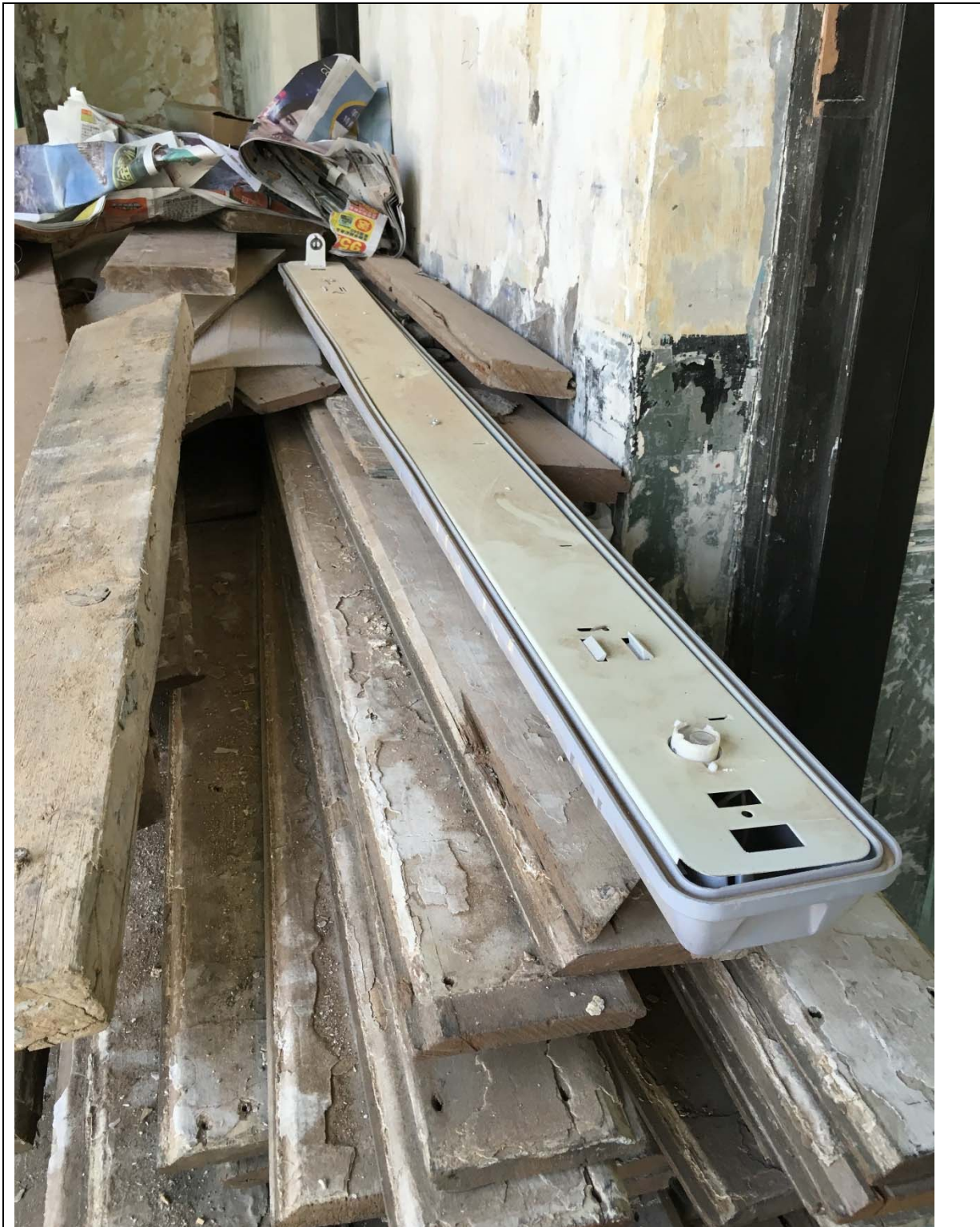
Above, photograph taken on 2 nd March, 2016, showing timber boarded ceiling was stored inappropriately with trashes.
