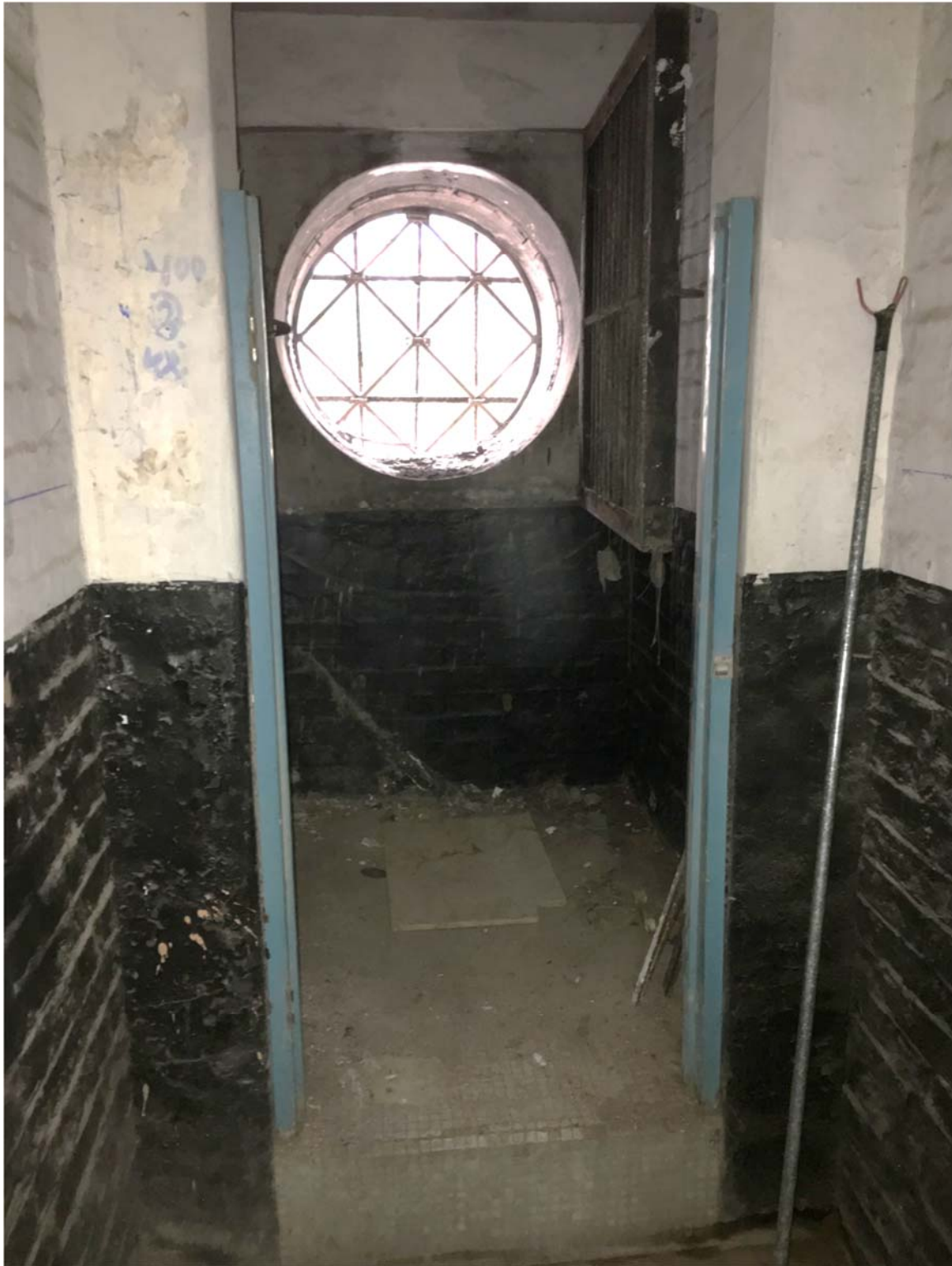
Above, photograph taken on 25 th February 2016, the conduits, lighting, mesh and fan on the window, timber panel door were incorrectly removed.
