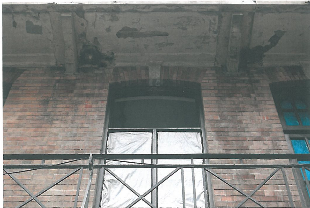
Above, photo taken on 18 th March 2016, showing spilt concrete on the Block 9 Magistracy West elevation (1/F).
