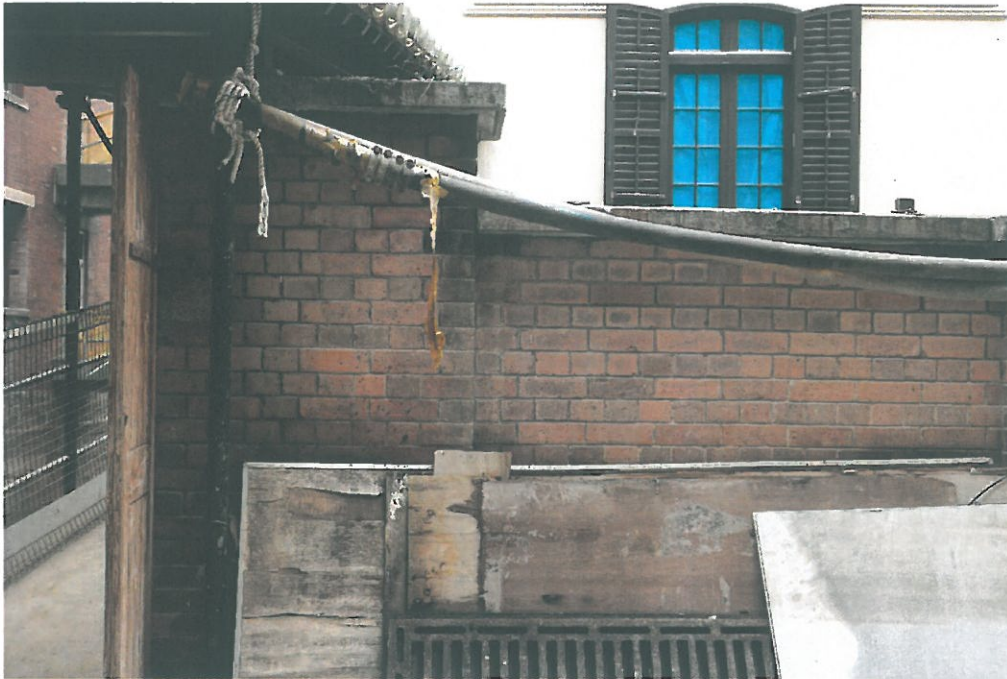
Above, photo taken on 18 th March 2016, showing spilt concrete on the boundary wall opposite Block 9 Magistracy West elevation.
