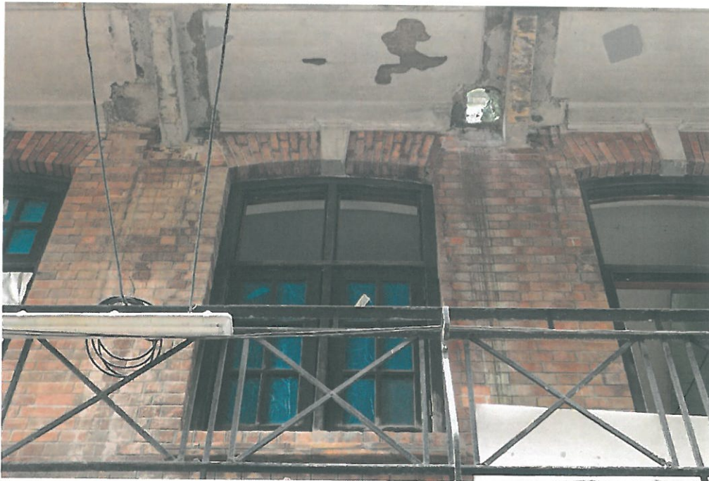
Above, photo taken on 18 th March 2016, showing spilt concrete on the Block 9 Magistracy West elevation (1/F).
