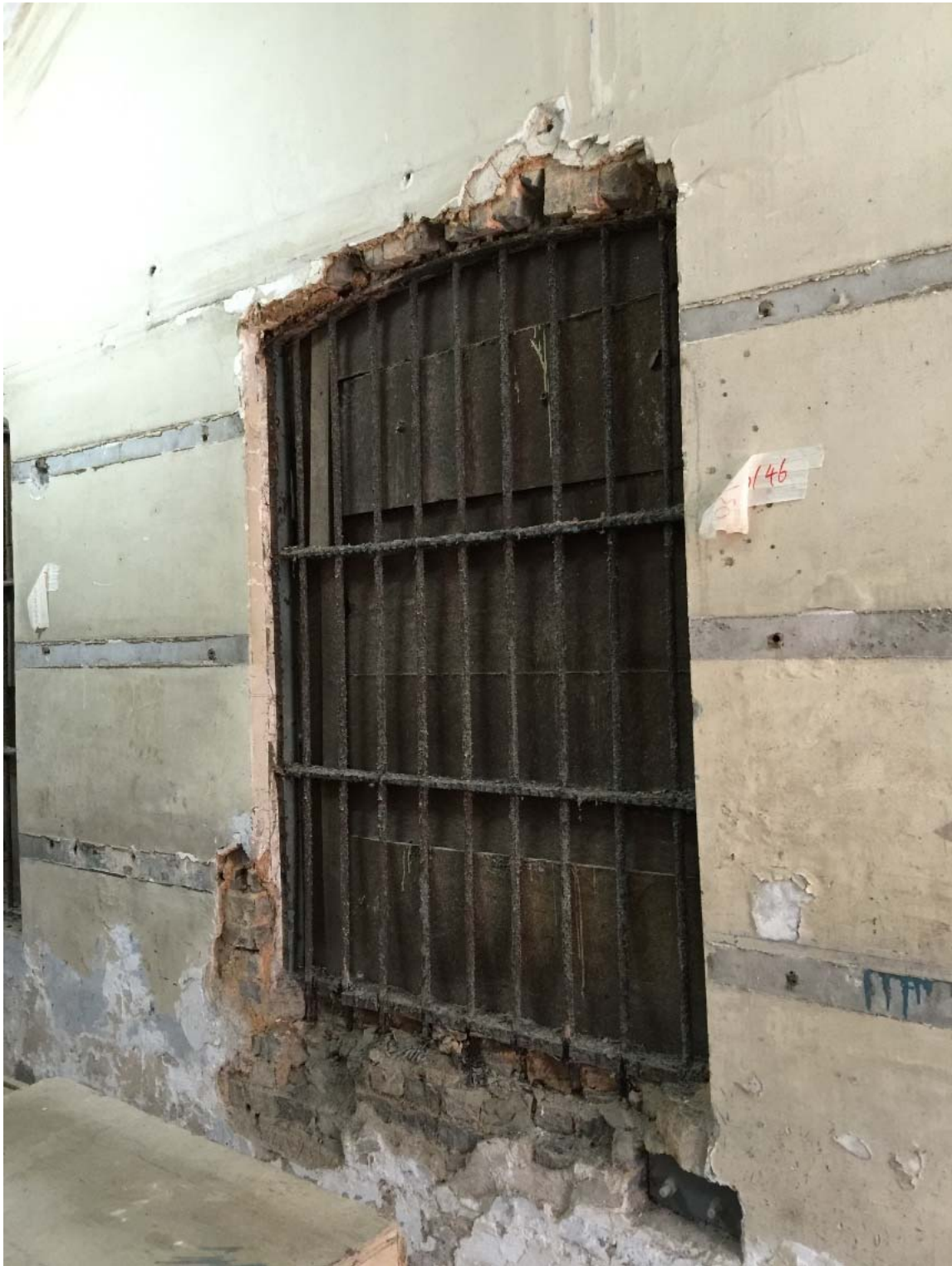
Above, photograph taken by the Management Contractor on 10 th March 2015, showing the metal bar screen.
