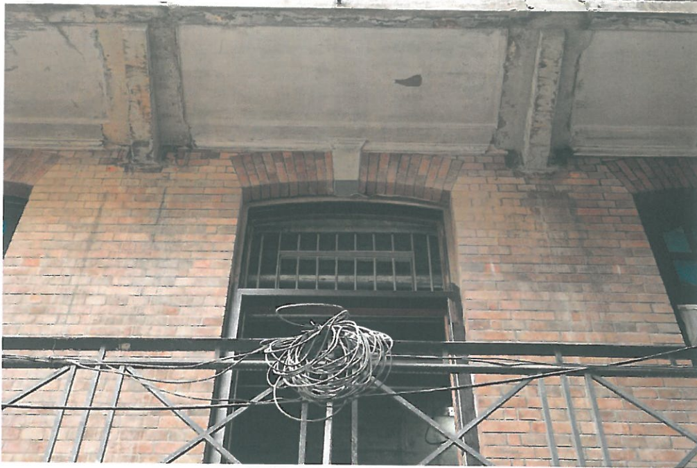
Above, photo taken on 18 th March 2016, showing spilt concrete on the Block 9 Magistracy West elevation (1/F).
