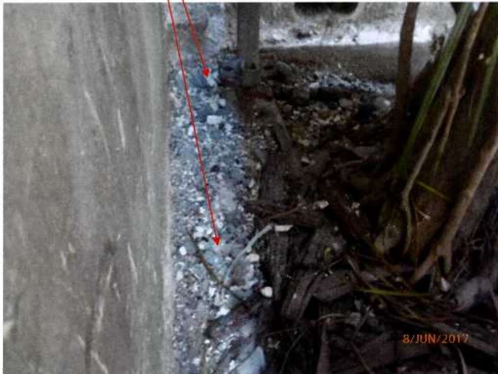
Fig. 3 Lots of construction debris scatter at the corner of the planter.
