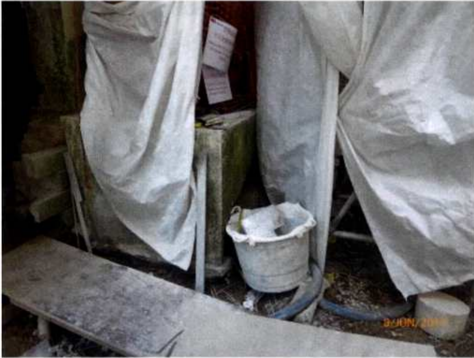
Fig. 10 Many construction materials are placed near the planter.
