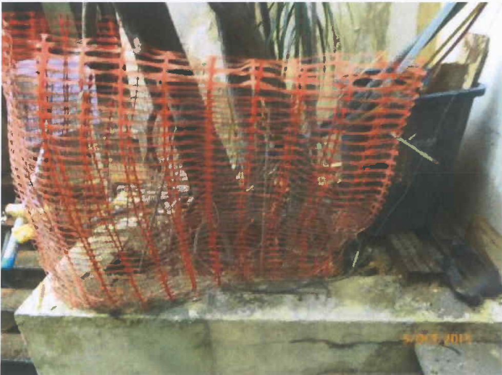
Fig. 9 The small cordon zone is not in order.
