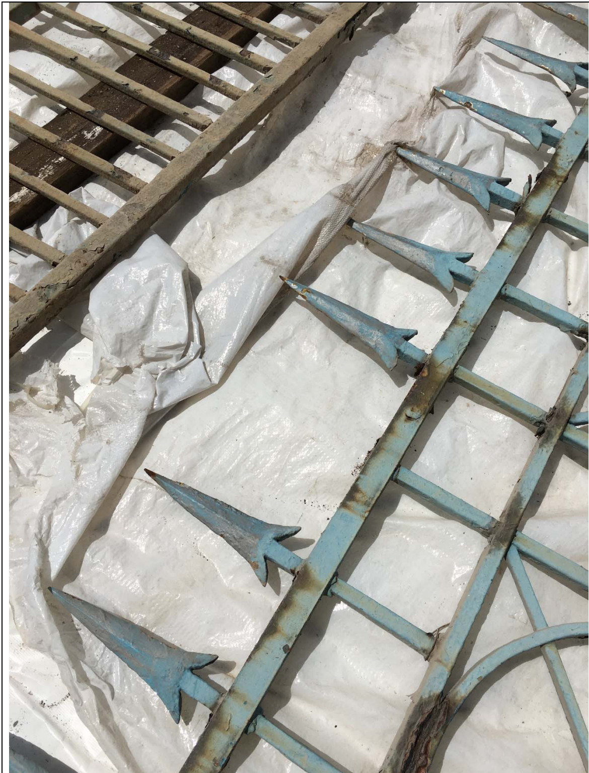
Above, photo taken on 21 st July 2016, showing one arrow on left hand side leaf was missing.
