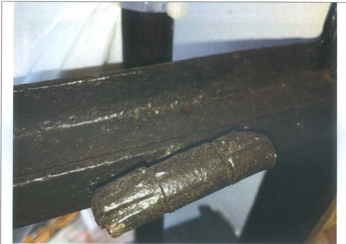
Above, photograph taken on 15 th July 2016, showing the casement was cut above the hinge.
