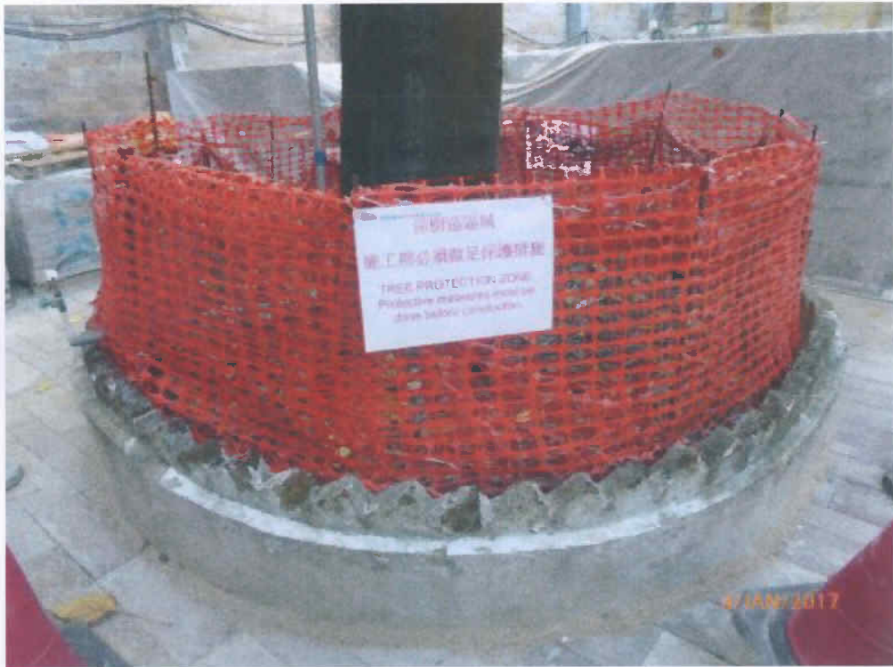
Fig. 10 We recommend to erect a Tree Protection Zone (similar to the following photo) at the planter especially during the nearby renovation works are in progress.
