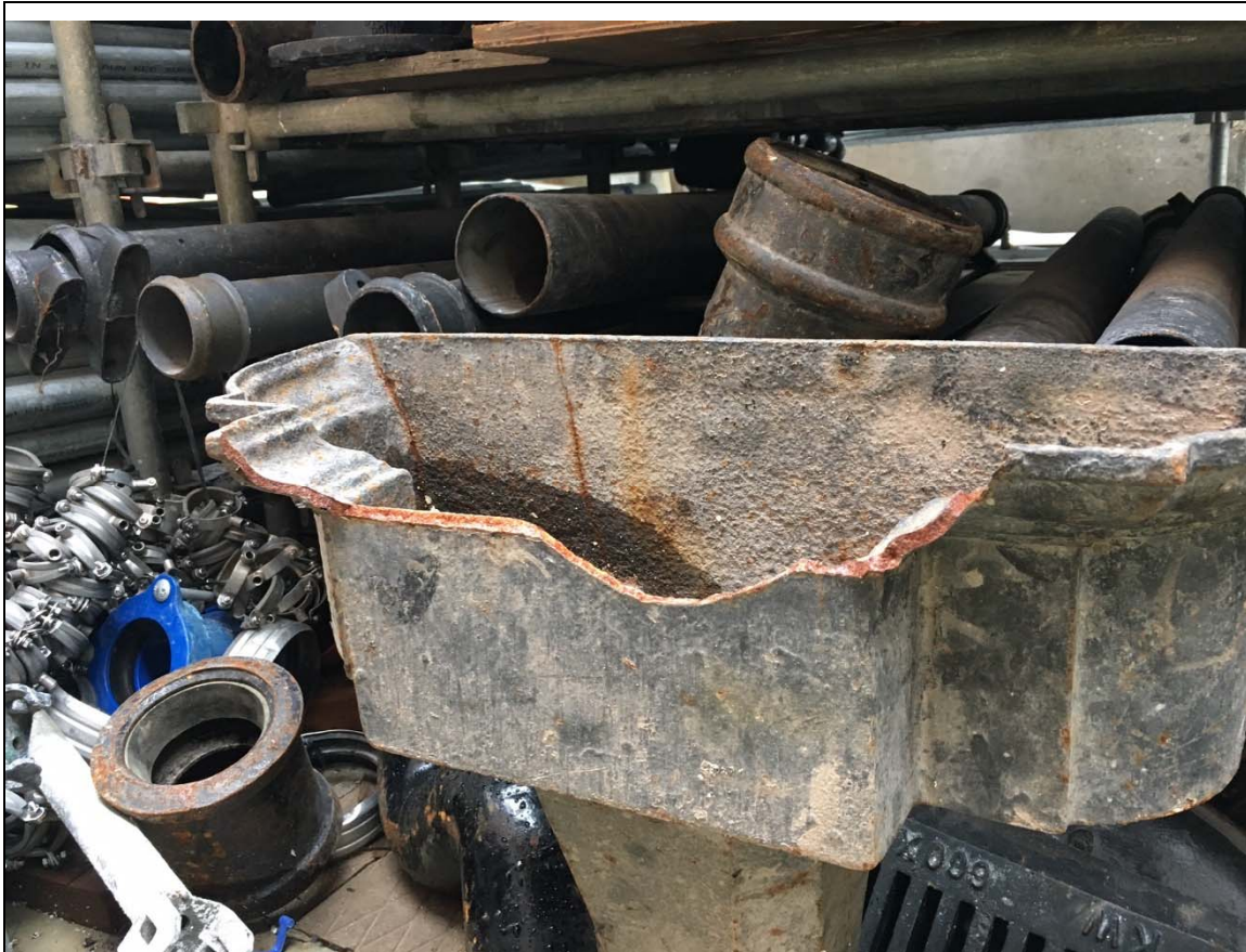
Above, photo taken on 27 th April 2017, showing the hopper was damaged.
