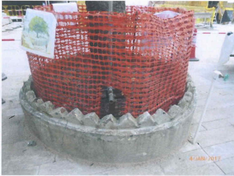
Fig. 10 We recommend to erect a Tree Protection Zone (similar to the following photo) at the planter especially during the nearby renovation works are in progress.
