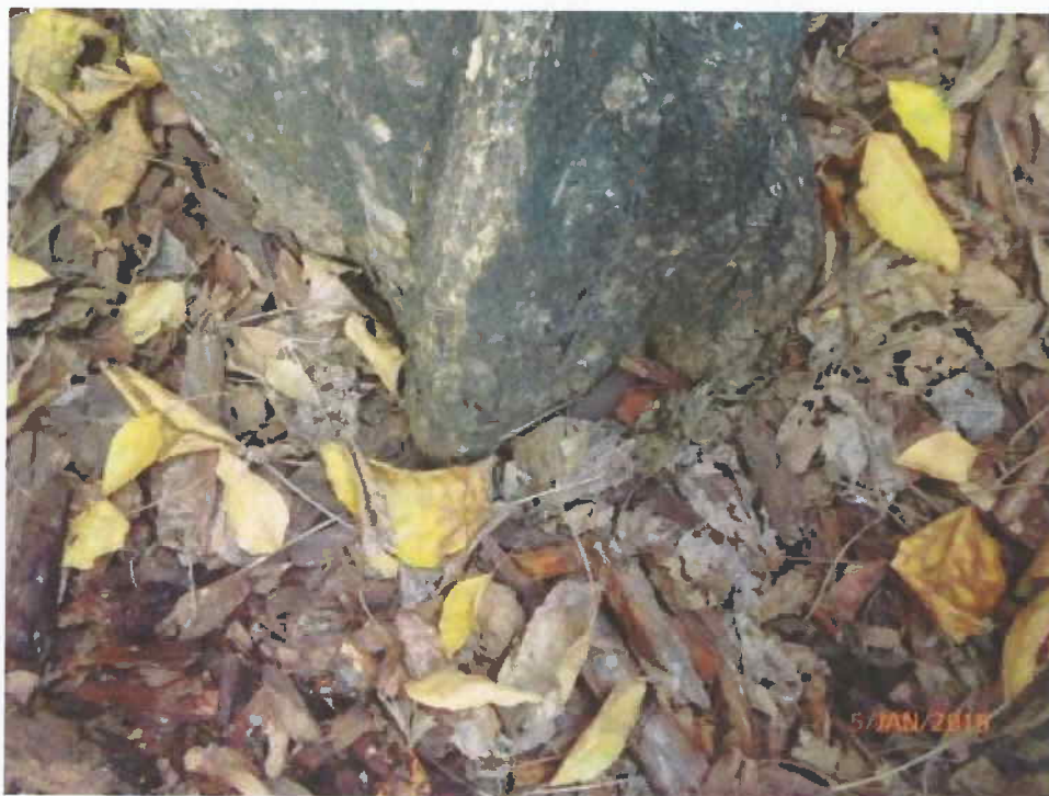
Fig 2. Root collar is normal. The planter is full of mulch and leaves.
