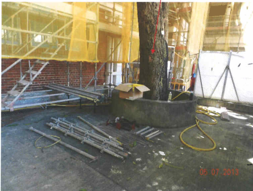
Fig. 3 Scaffolds have been set up inside the cordon zone. Many metal tubes are placed near Tree-5. Some wounds are found on the lower trunk.
