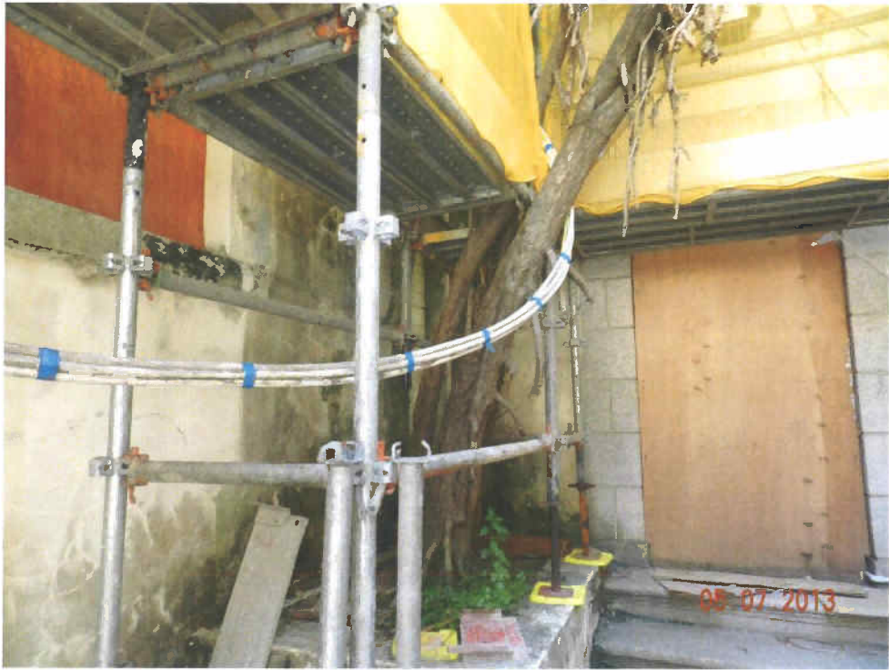
Fig. 4 A scaffold has been set up at the planter for further renovation of the nearby building.
