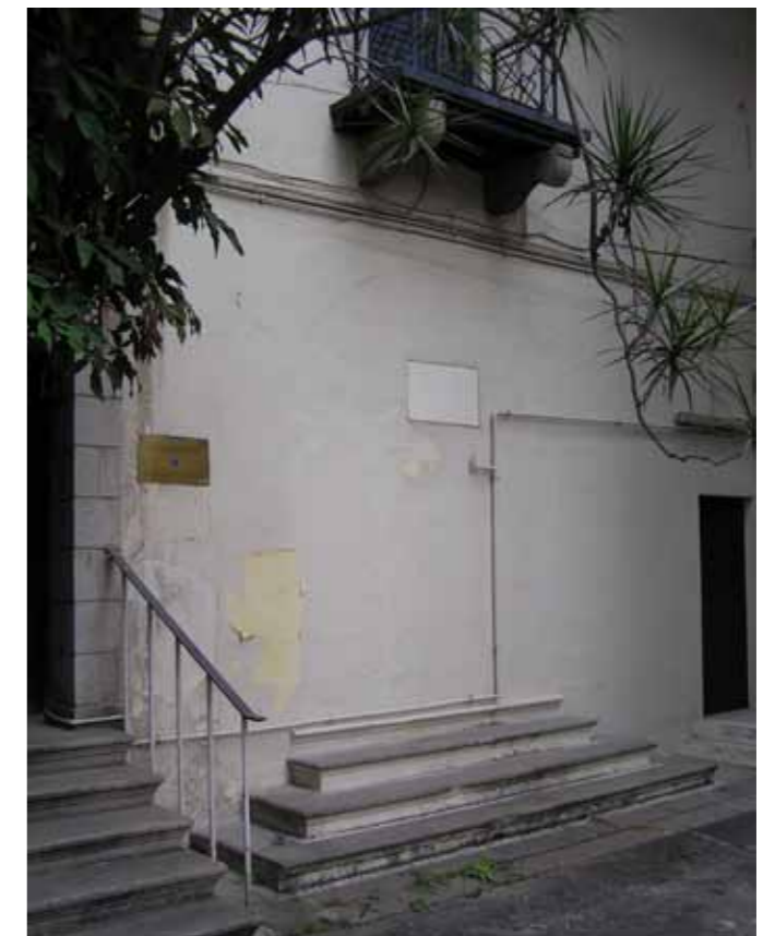
Figure 5 - Large archway on east wall which was early prison entrance but has since been blocked
