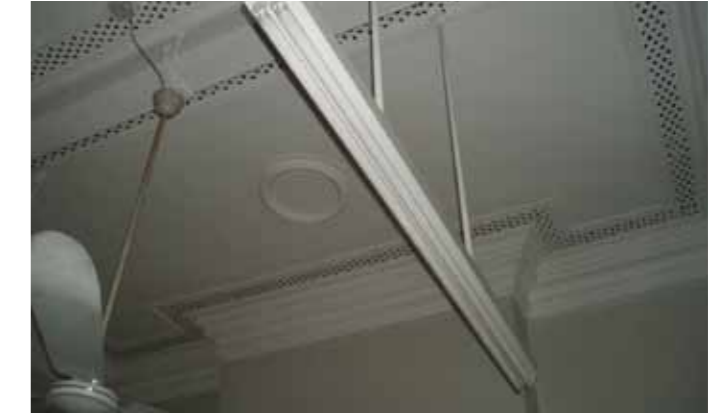
Figure 8 - View of the ceiling in the second floor Married Inspector's Quarters (west block)
