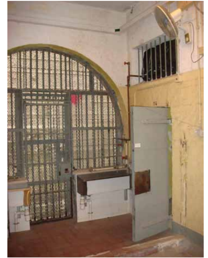
Figure 9 - The ground floor archway at the west end of the building. Note the later door on one of the cells and the sinks installed at an unknown date.
