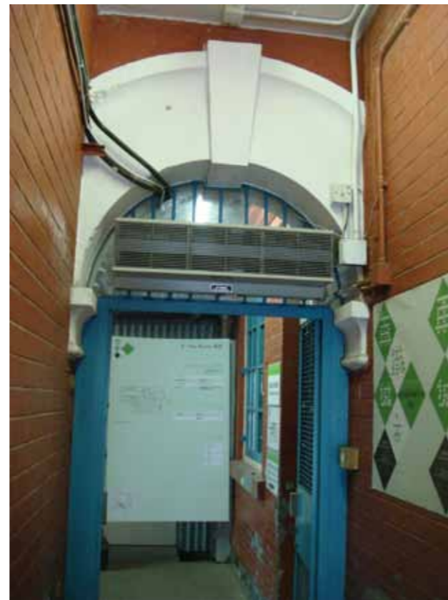
Figure 6 - Archway at the west end of the ground floor, which leads through to the prison.
