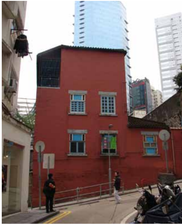
Figure 1 - West elevation as viewed from Staunton Street. Various alterations to the windows can be seen.
