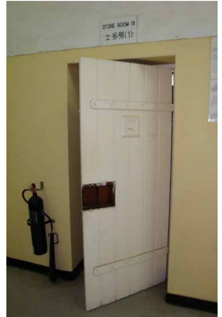
Figure 13 - One of a few timber doors in the west wing second floor
