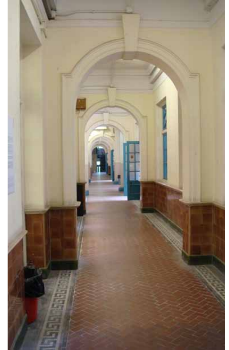
Figure 8 - The ground floor corridor with decorative keystone arches, Canton tile floor with Greek key border and glazed tiled dado
