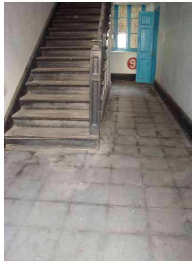
Figure 11 - View of the ground floor of the Deputy Superintendents' House (east block) staircase
