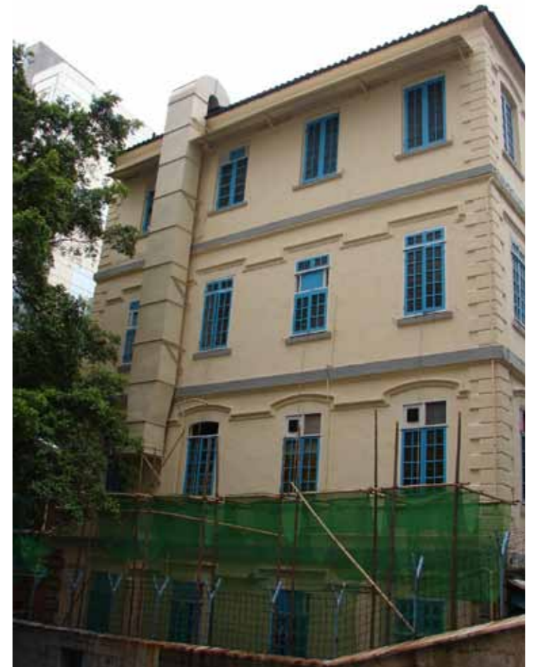
Figure 4 - West elevation showing large ductwork for one of the modern kitchens and third floor corrugated metal sunshade
