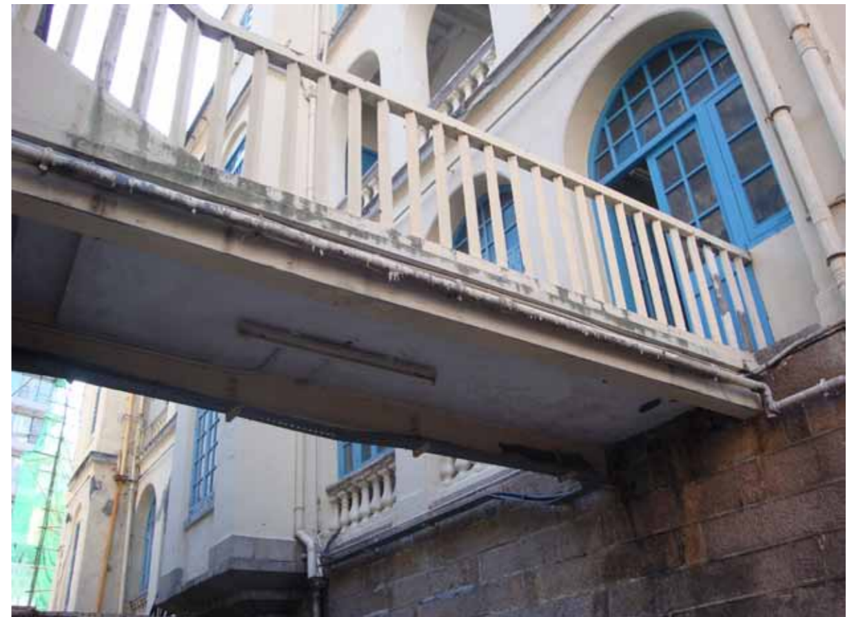
Figure 4 - Link bridge between the north side of Building 04 and the south side of Building 06
