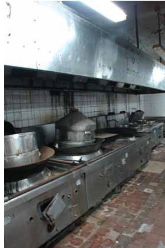
Figure 7 - Large cooking equipment in the first floor kitchen
