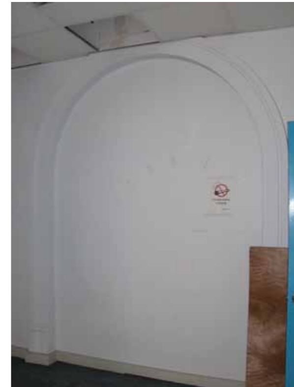
Figure 10 - Blocked archway in 02/G/03
