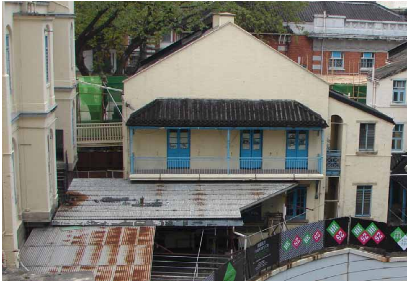
Figure 1 - East elevation of the building. The corrugated iron coverings have been partially removed since this photograph was taken.
