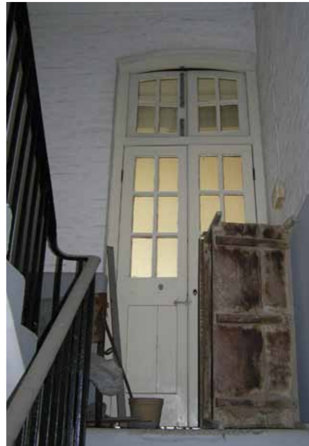
Figure 19 - Doors in the secondary stair at the south end of the building
