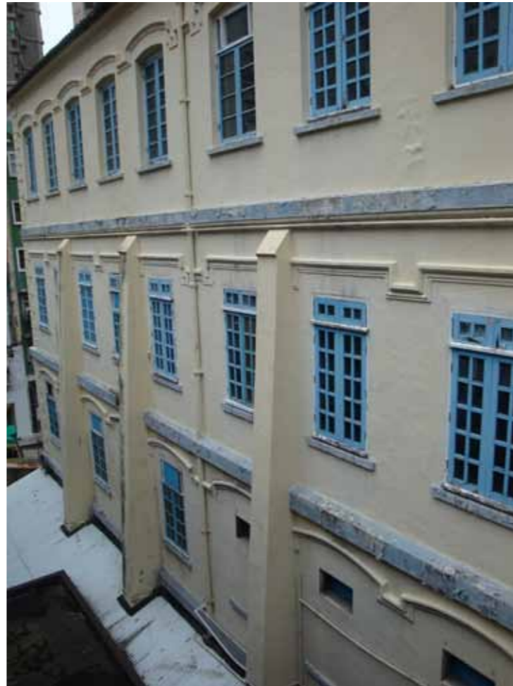
Figure 3 - Partial view of the south elevation showing blocked windows on the ground floor, and buttresses added c.1906
