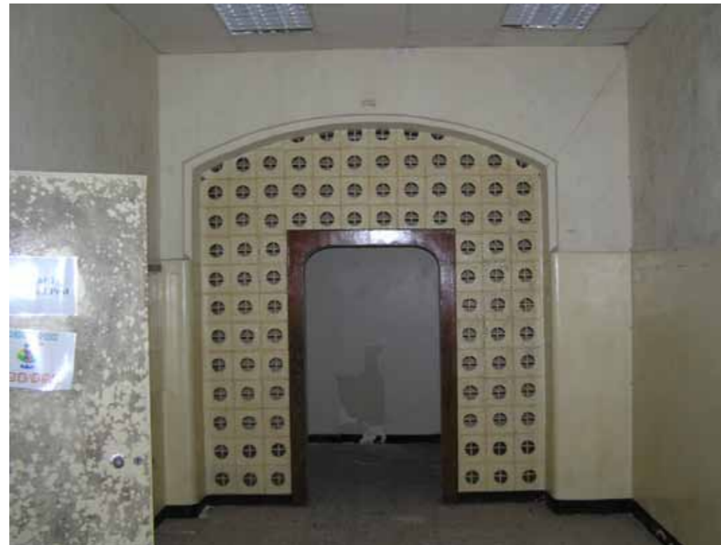
Figure 10 - Blocked ground floor arch which would have been the west end of the prison entrance pre-1930s
