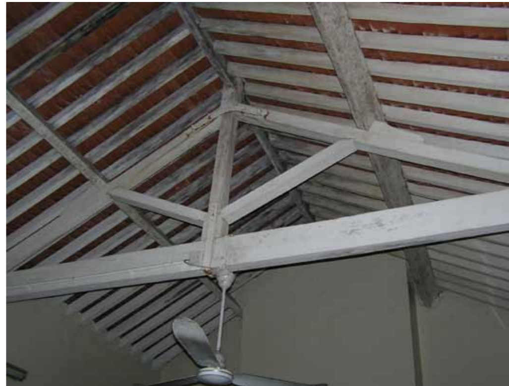
Figure 15 - Timber frame roof structure visible on the first floor of the southwest extension
