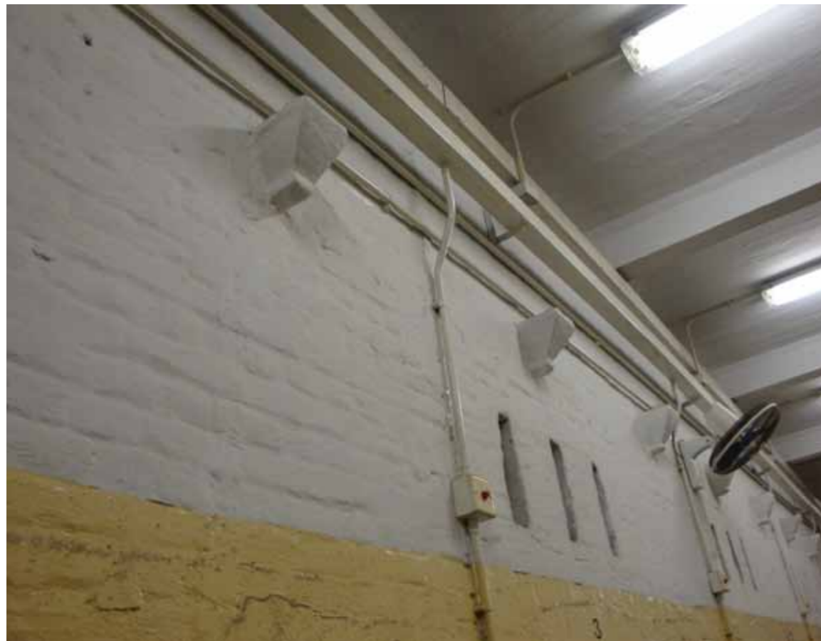
Figure 7 - Corbels in the west wing first floor which indicate the original level of the ceiling
