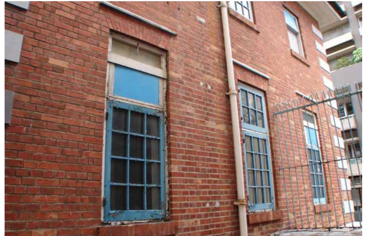
Figure 3 - Windows on the south elevation. The ground floor central window has the original/early casement with fanlight casement above, while those either side have been altered to accommodate air conditioning units.
