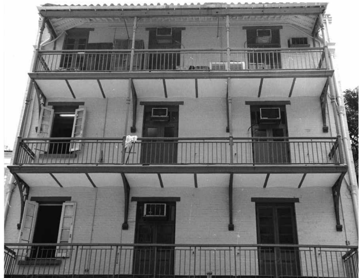
Late 20th century photograph (exact date not known) of the north elevation showing the ground floor balcony still in place and air-conditioning units installed.
