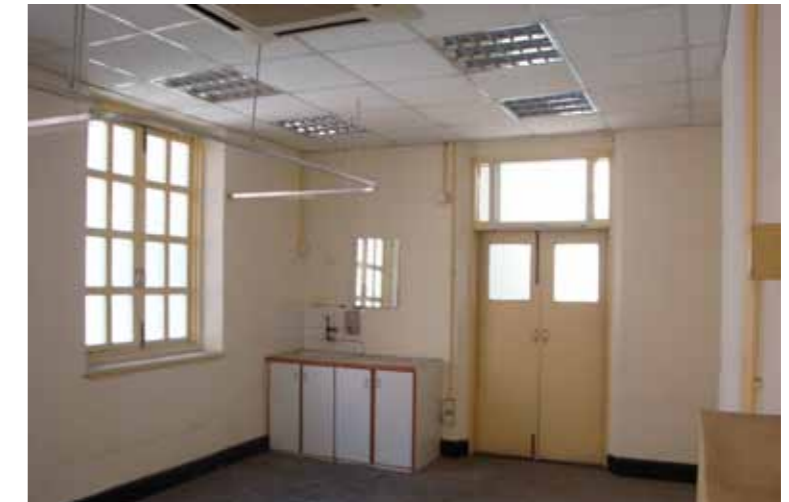
Figure 5 - Typical interior space, with later suspended ceilings and replacement double doors. The fanlight has been altered to accommodate air-conditioning.
