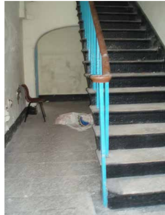
Figure 12 - View of the ground floor of the Married Inspector's Quarters west entrance hall
