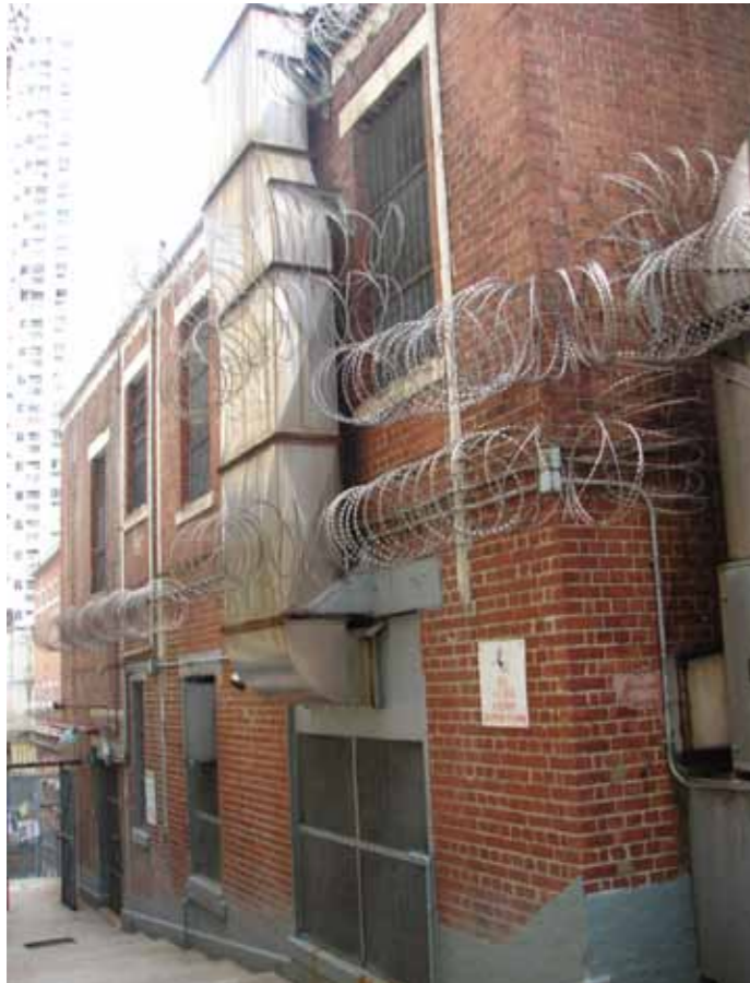
Figure 1 - Exterior view of the south elevation, showing a large exhaust duct from a kitchen window
