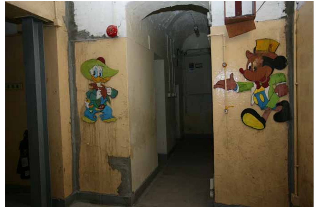
Figure 21 - Remnants of use as a paediatric ward on the second floor of the east wing
