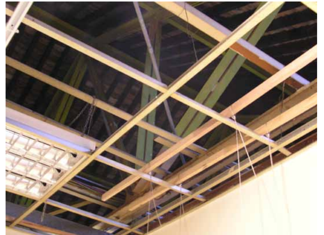
Figure 15 - Steel truss roof structure. The lower grid is the modern inserted ceiling. The original ceiling is above the rafters.
