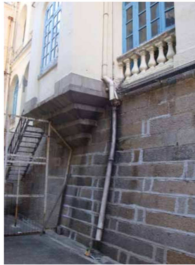
Figure 6 - Granite corbel supporting one of the north projecting bays. The other is in need of urgent repair.
