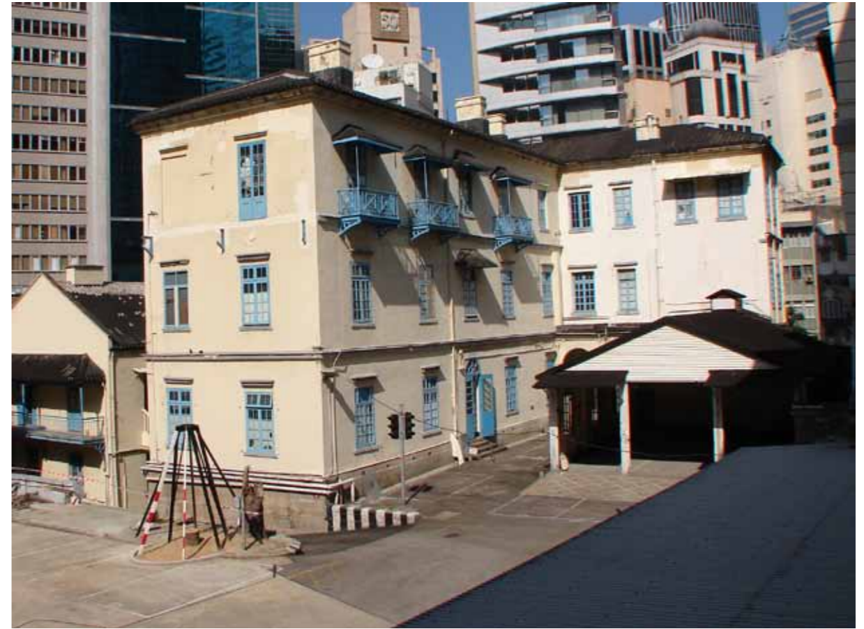
Figure 2 - Southwest elevation; note the missing balcony on the west end, second floor
