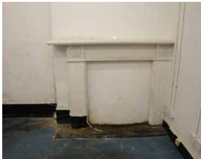
Figure 8 - The last surviving fireplace in the building, in one of the ground floor west rooms
