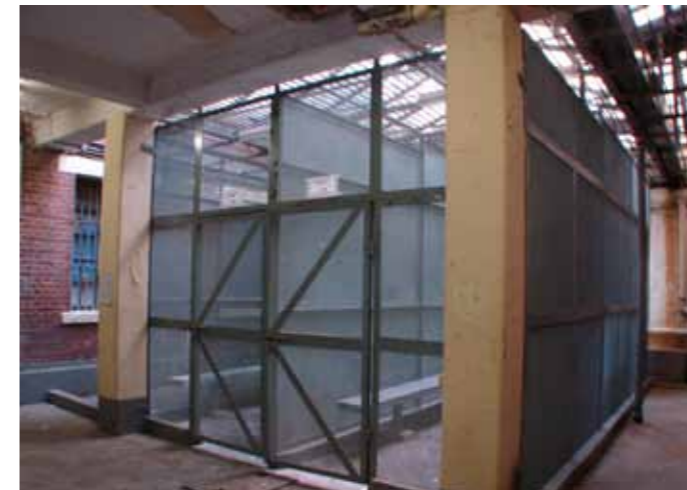
Figure 12 - Cells on the ground floor which have been constructed within the lightwell
