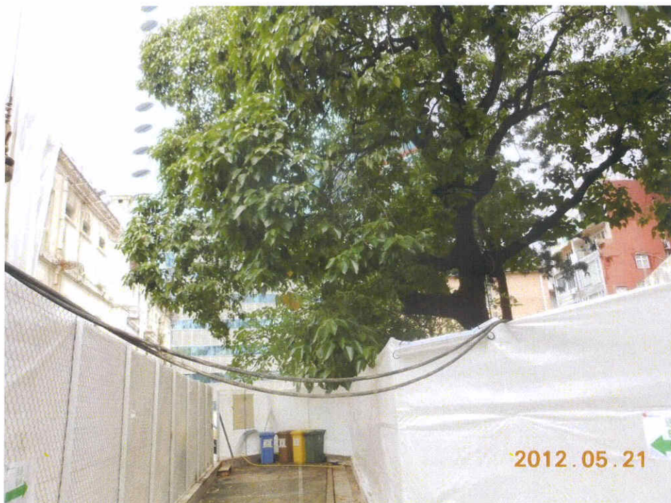
Fig. 5 Overgrown branches /leaves were too close to the fence of the cordon zone during the inspection on 21 st May 2012.
