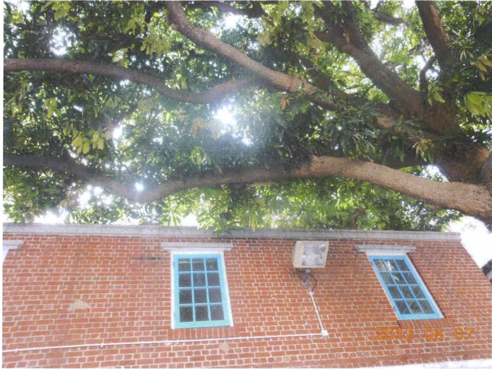
Fig. 4 Some lower branches and leaves are too close to the nearby buildings. Trimming of such branches/leaves is recommended.
