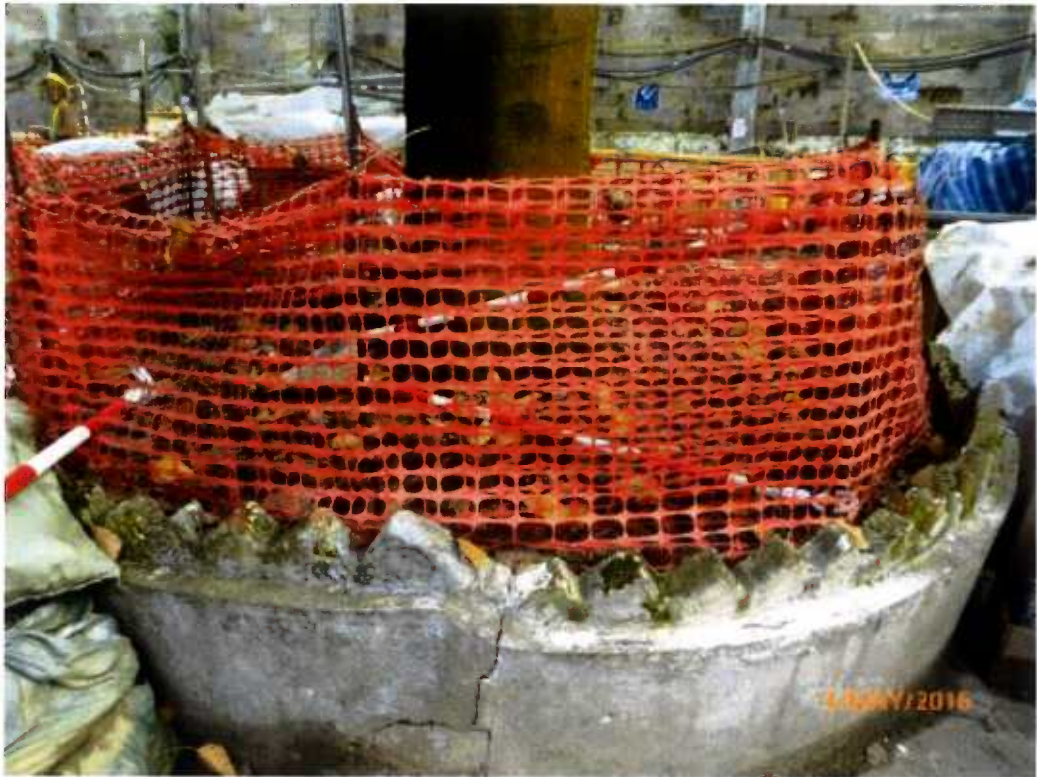
Fig. 10 The small cordon zone is in good order at the time of inspection.
