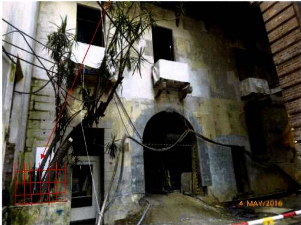
Fig. 9 Renovation works are in progress near Tree-11. Recommend to set up a small cordon zone to protect the tree.
