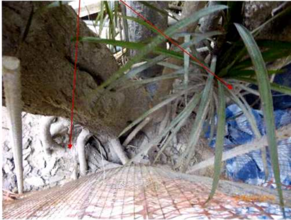
Fig. 2 Lots of cement dust are still found on the planter.
