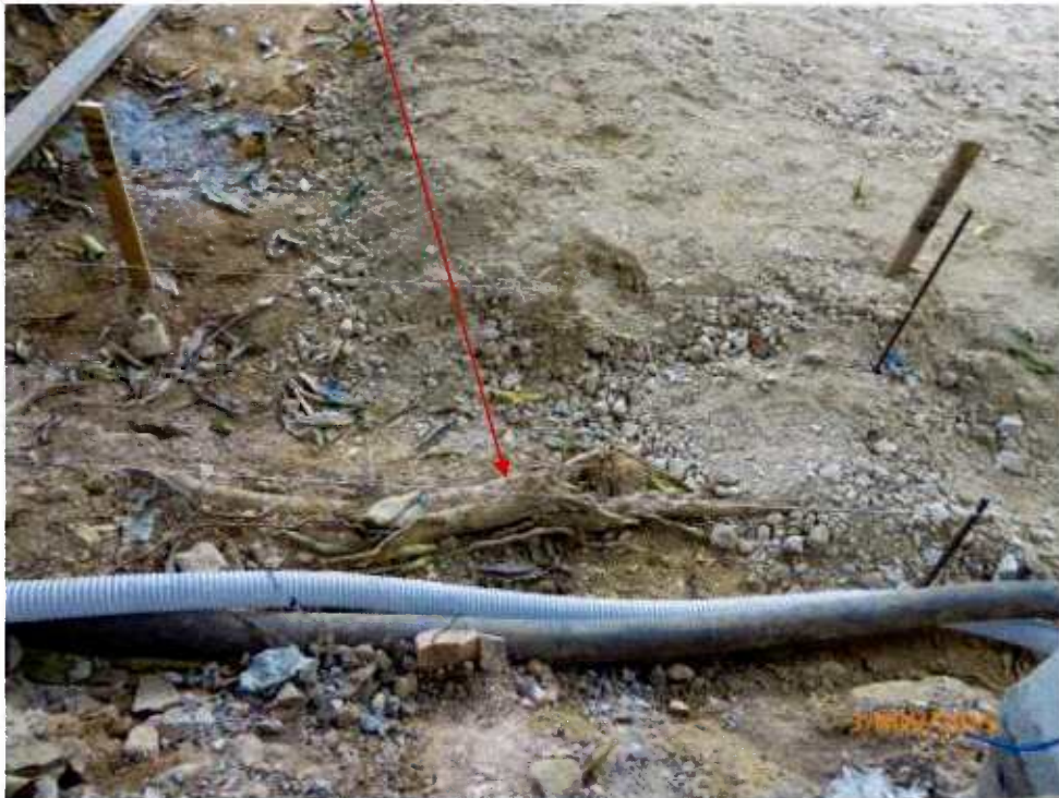
Fig. 9 A large bare root has exposed on ground surface. More protection work for this root is recommended.
