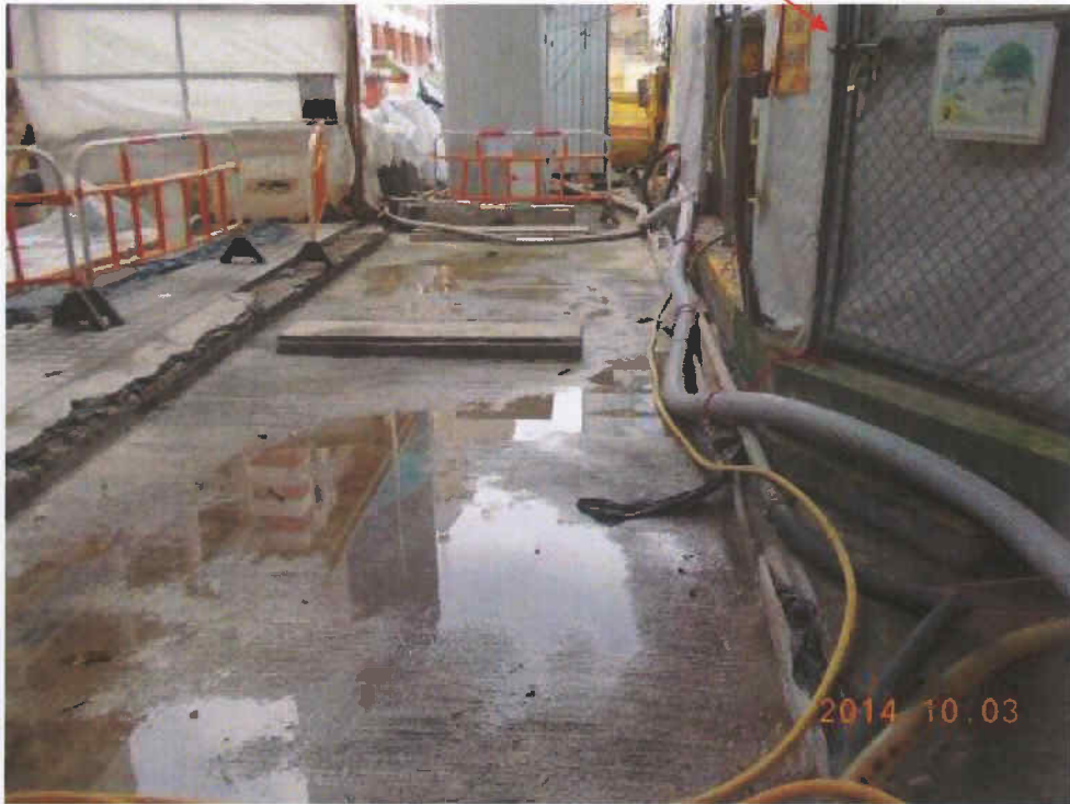
Fig. 8 Cleanliness of the site near the entrance is acceptable.
