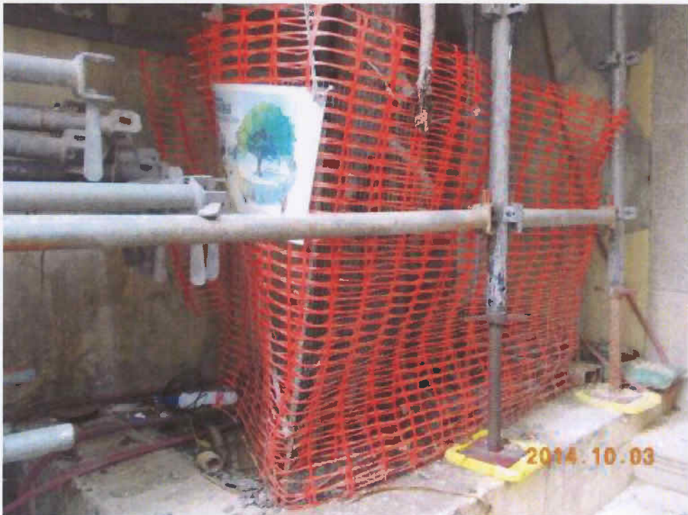
Fig. 9 The small cordon zone has been broken by the metal tubes.
