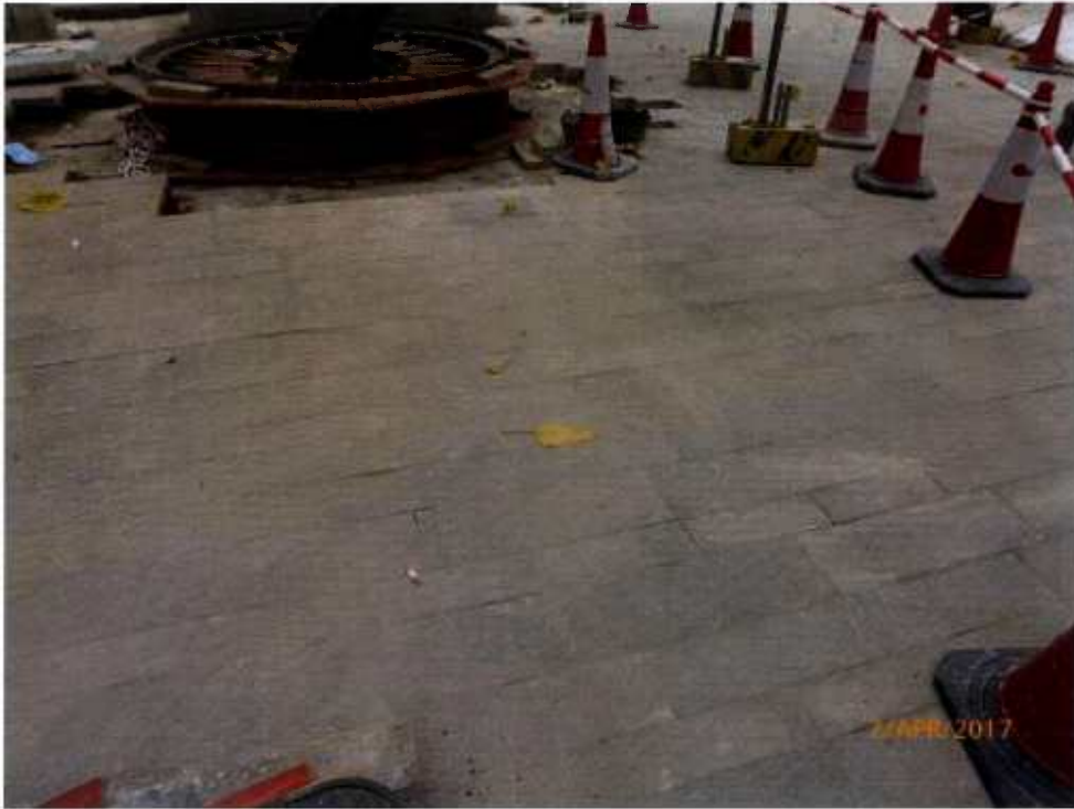
Fig. 8 The planter is under repair.
