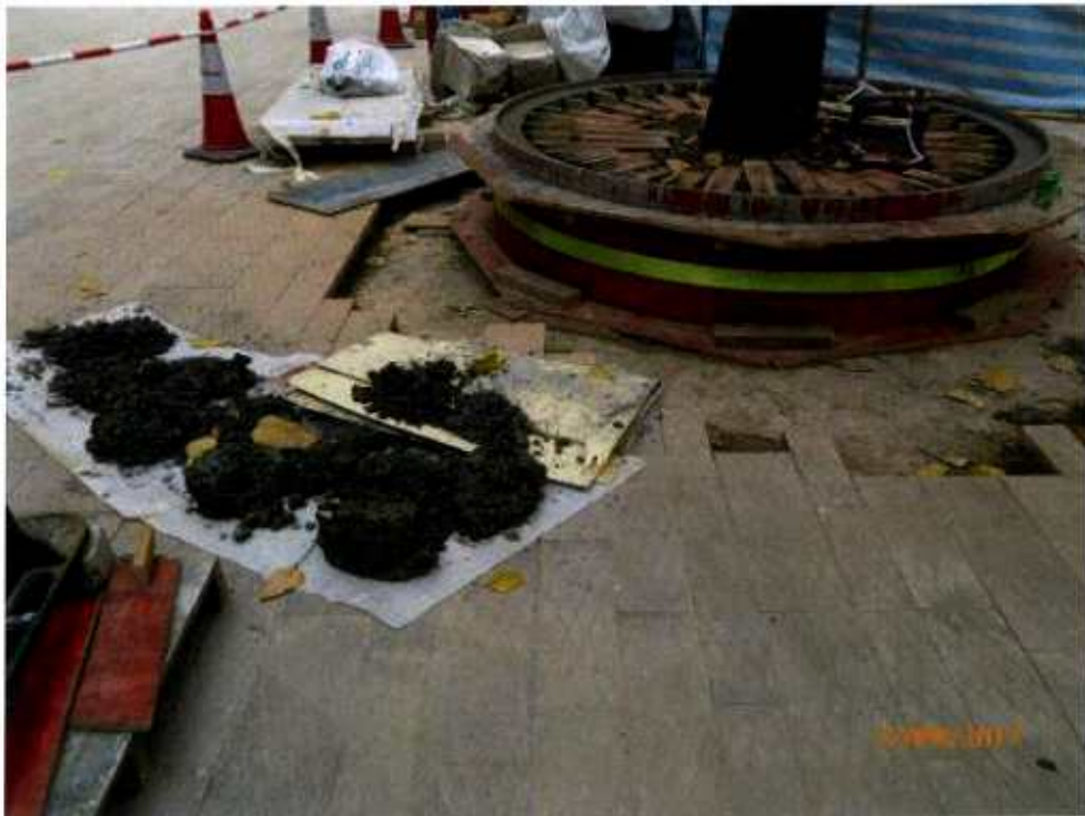
Fig. 9 The planter is under repair.
