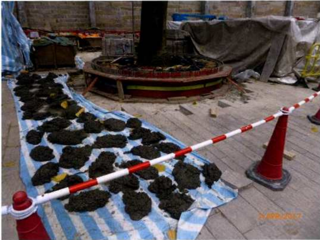
Fig. 10 Many construction materials are placed near Tree-6.
