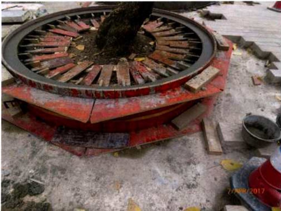
Fig. 7 The planter is under repair.
