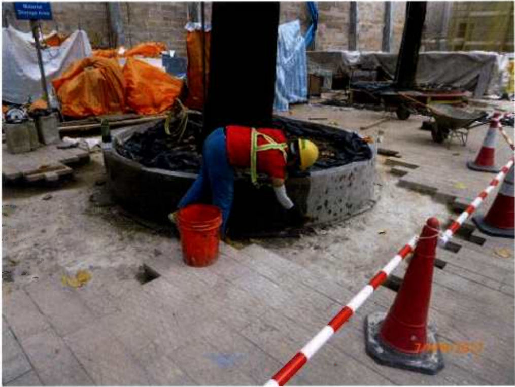
Fig. 10 The planter is under repair at the time of inspection.
