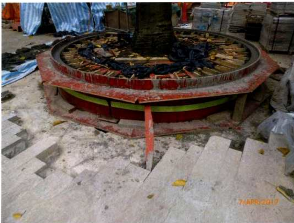
Fig. 9 The planter is under repair at the time of inspection.
