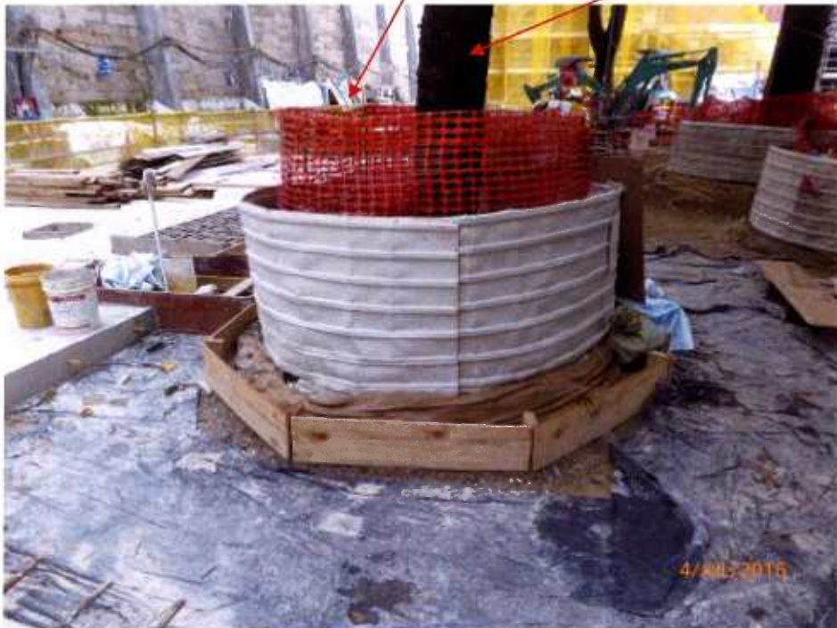
Fig. 3 Recommend to set up a small cordon zone (similar to Tree-9) to protect the tree.
