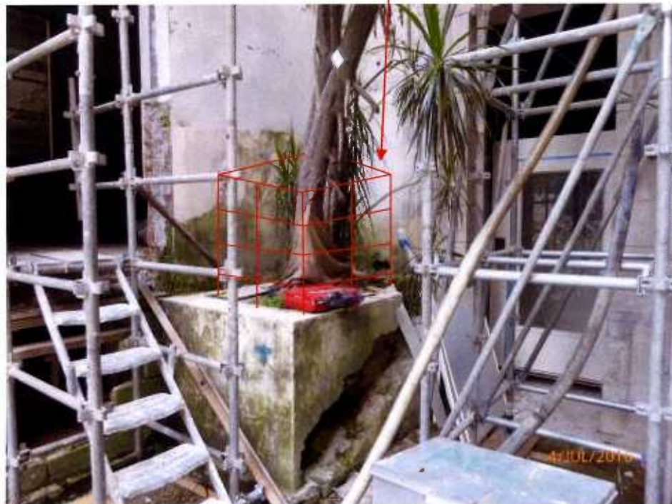
Fig. 3 Recommend to set up a small cordon zone to protect the tree.
